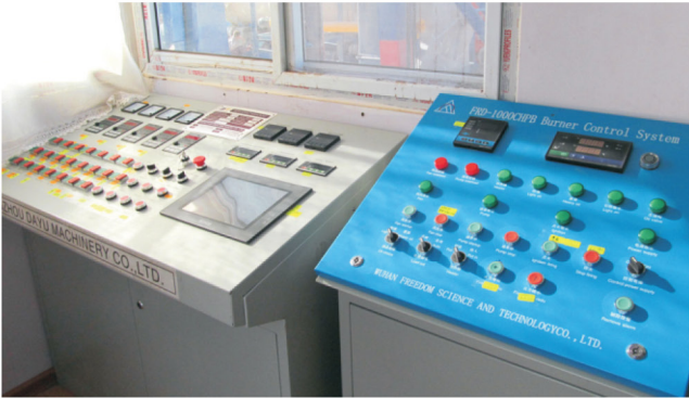
Sistema de control Electrical control system
